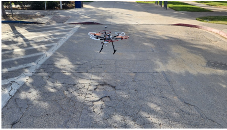
Fig. 7: Experiments conducted to detect faults in the road using the prototype quadcopter drone.
